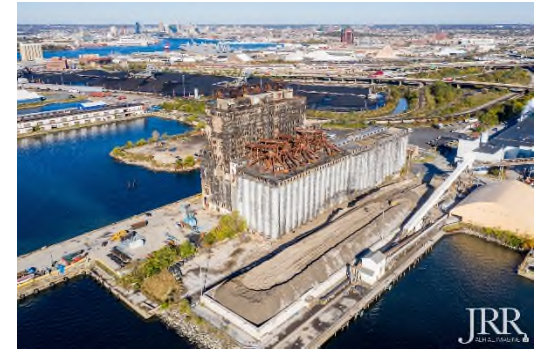
Pier 13, Baltimore, MD Building Height: 210 ft. Demolish former grain silo and associated offices using ultra-high reach demolition tool and a 140-ton crane.
