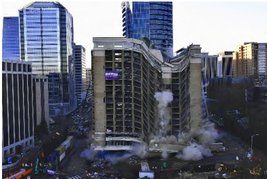
Holiday Inn Rosslyn, Arlington, VA Mechanical demolition of a parking garage and pedestrian bridge. Implosion of an 18-story hotel.
