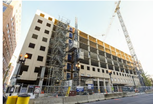
20 Massachusetts Avenue, Washington D.C. Asbestos abatement, strip out, façade removal, and roof strip of an 8-story office building.
